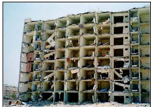
Figure 1.12 Khobar Towers Bombing, Dhahran, Saudi Arabia; Casualties from Debris, Not Collapse
