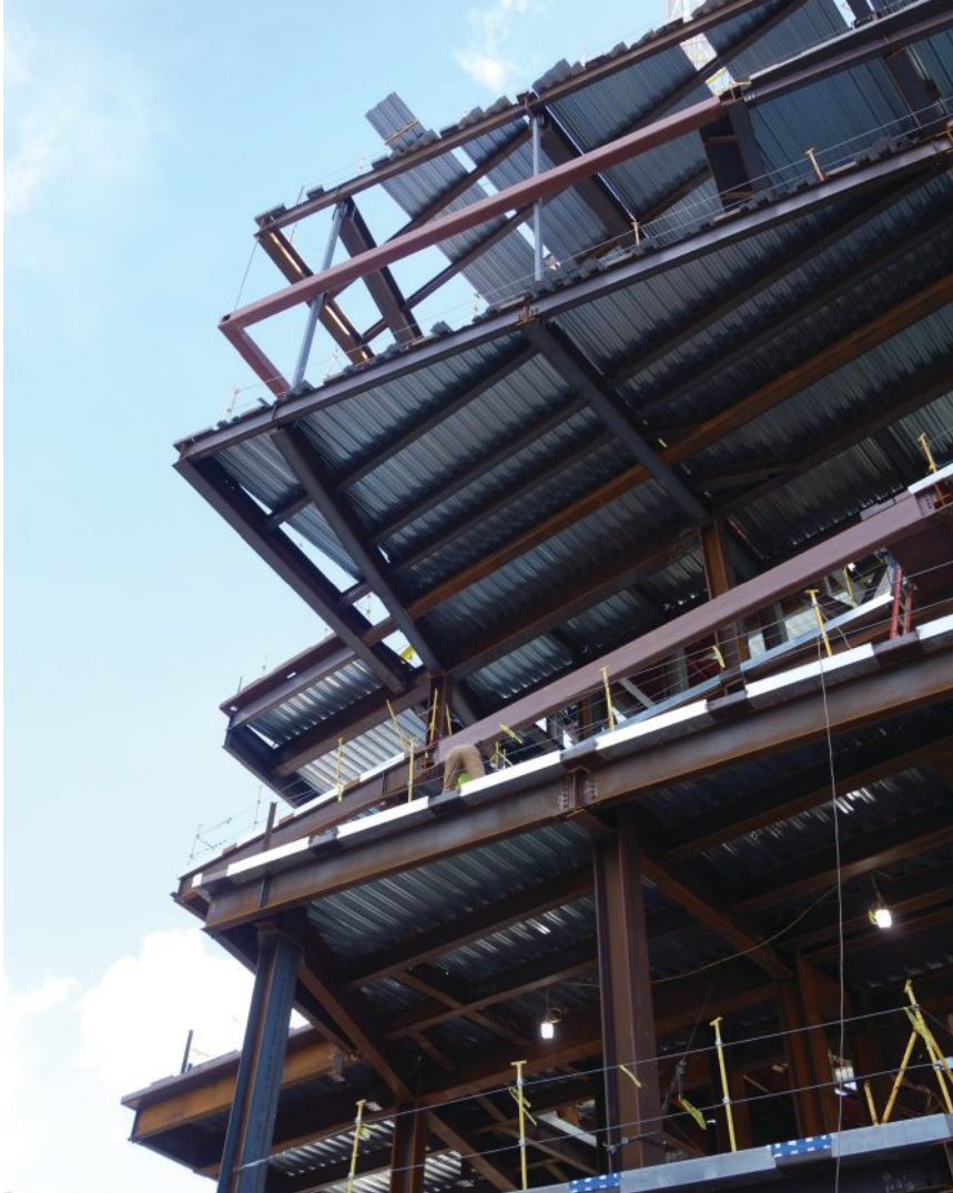
At Level 7's northwest corner (pictured), two W36x487 girders cantilever west and create a 25-ft overhang. .....
