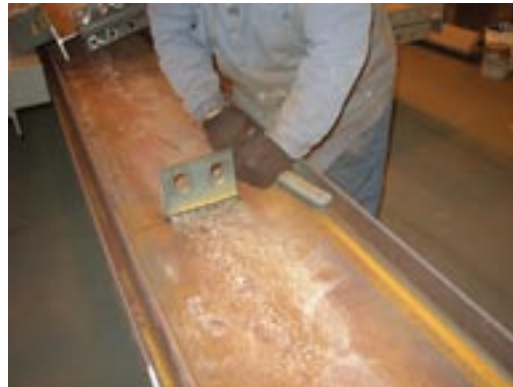
A worker uses a wire brush to prepare a member to SSPC-SP2. Photo courtesy of Atlas Iron Works, St. Louis.
