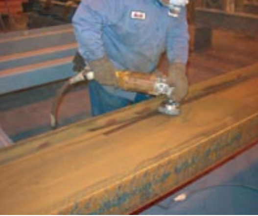
A worker prepares a member to category SSPC-SP3. Photo courtesy of Atlas Iron Works, St. Louis.
