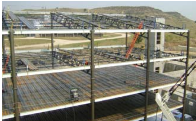
Figure 2: Reclaimed Pipe columns at the NREL Laboratory in Golden, Colo. Courtesy of KL&A Engineers.
