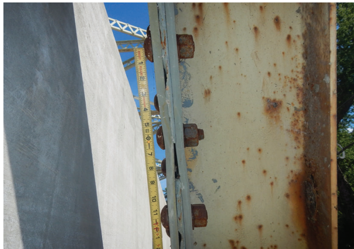
Figure 3-9—Plating repair with severe section loss and inadequately prepared irregular surface
