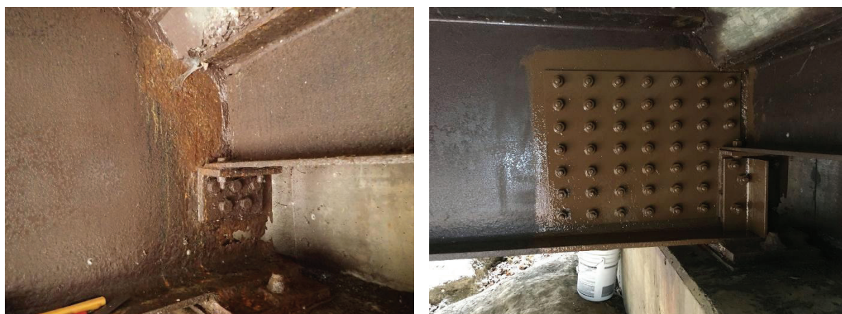
(a) Beam end with through-thickness section loss
