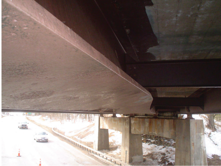
Figure 5-14—Impact damage to an interior steel girder of a multi-girder bridge
