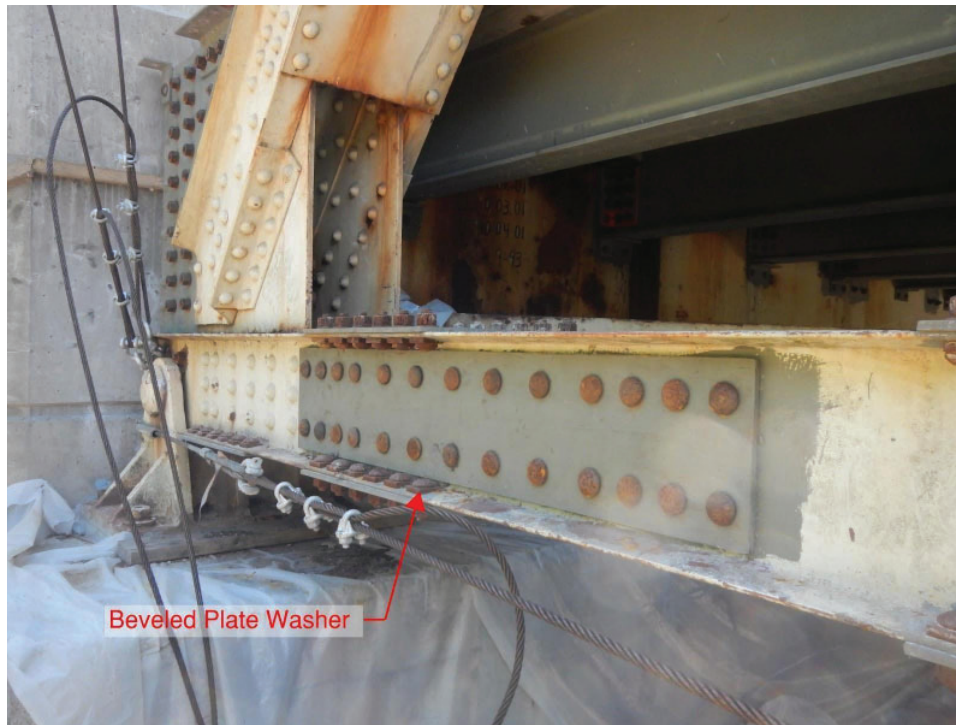
Figure 2-1—Truss bottom chord plating repair showing button-head bolts and beveled plate washers
