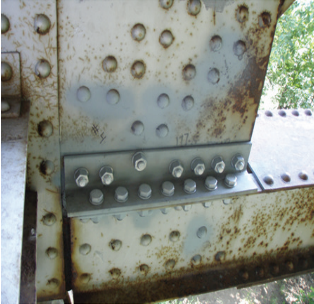
Figure 3-26—Localized angle repair to address section loss along the horizontal shear plane
