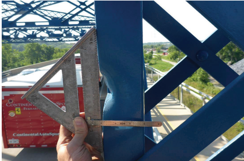
Figure 5-1—Local distortion of the projecting flange of a channel section used in a truss vertical member
