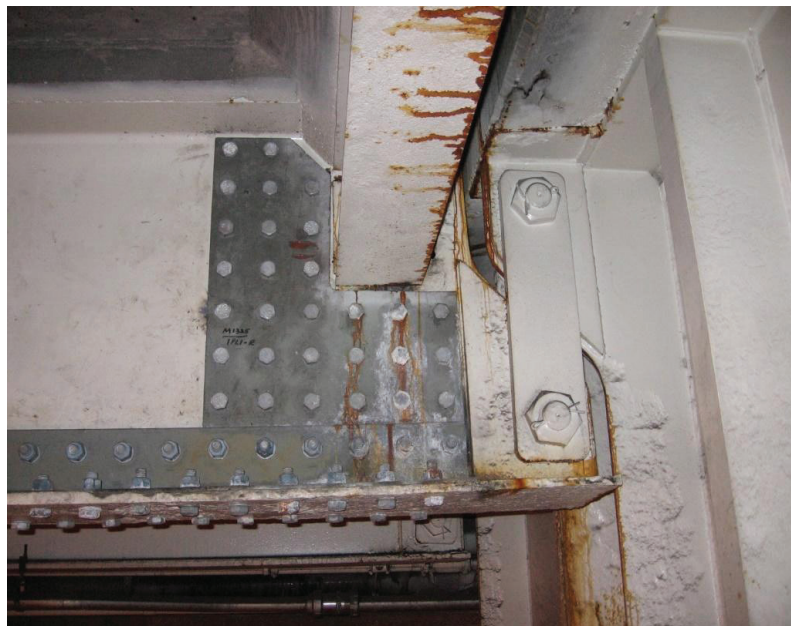
Figure 3-50—Plate strengthening repairs to address section loss of a girder web and flange adjacent to a pin and hanger connection
