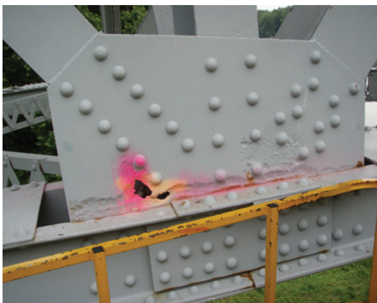
Figure 3-14—Gusset plate connection with severe pitting and through-thickness loss along the horizontal plane located just above the truss bottom chord
