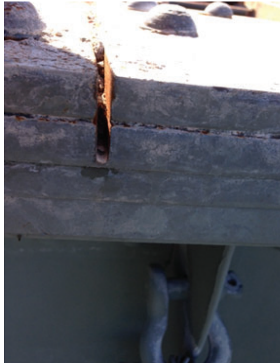
Figure 7-4—Saw-cut damage in a built-up top flange causing severing of the top plate and near-full section loss of the second plate from the top
