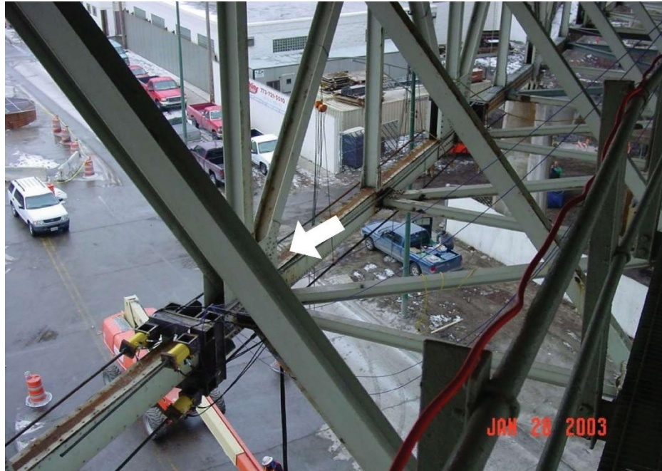
Figure 3-33—Supplemental tie rods to remove the existing load in the truss tension chord (arrow indicates gusset plate being repaired)
