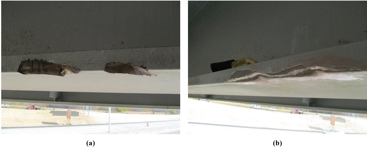
Figure 5-2—Gouging in a girder bottom flange (a) as discovered and (b) after grinding repairs
