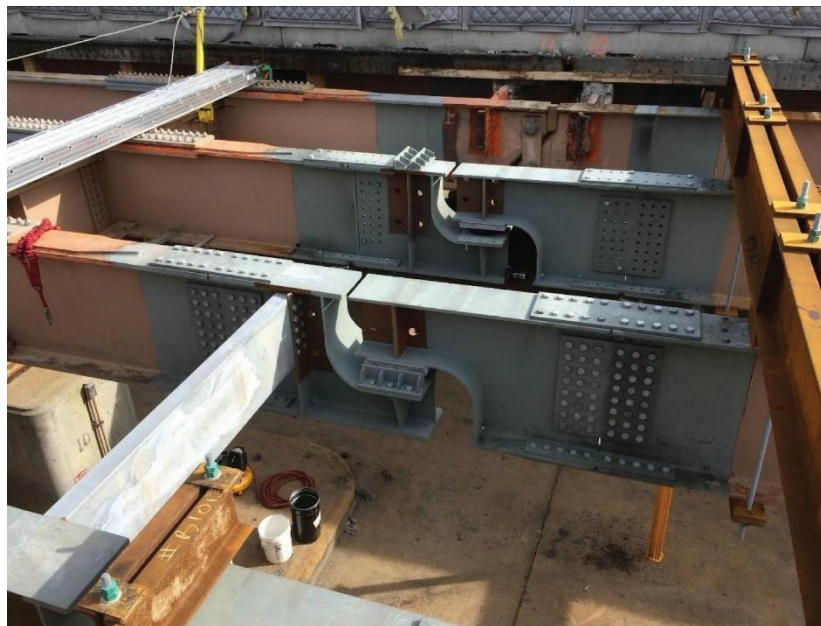
Figure 3-54—Example of a pin and hanger assembly replaced with seated beam connection (Linzell et al., 2017)
