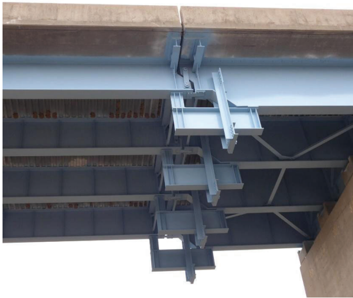
(a) Catcher beam for a bridge girder
