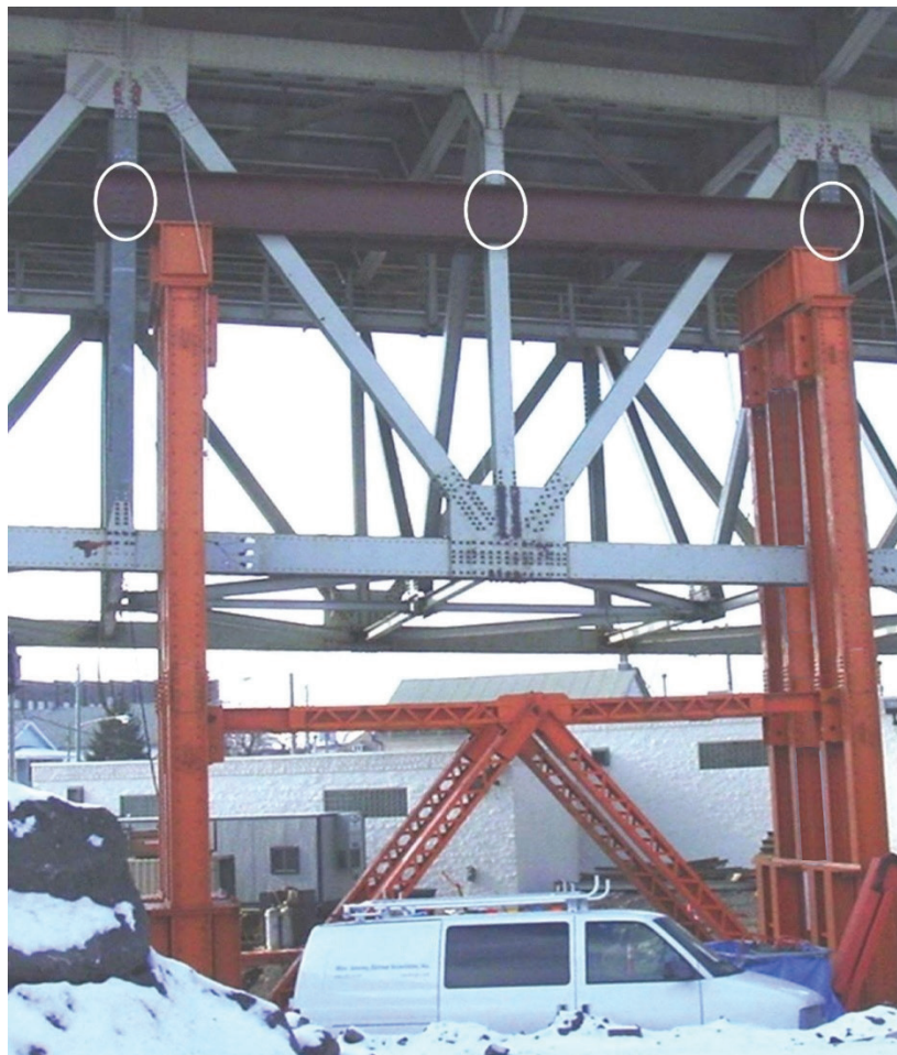
Figure 3-35—Example of supplemental truss shoring to perform a gusset plate replacement; circles indicate bolted connections for temporary truss support on the shoring tower header beam
