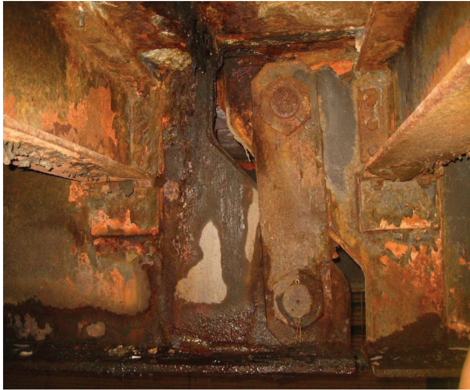
Figure 3-45—Severe corrosion of a pin and hanger connection that may create unintended torsional stress on the pin
