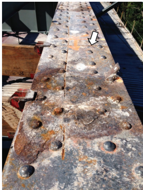
Figure 7-3—Example of a longitudinal saw cut in a built-up girder flange; arrow indicates a transverse saw cut
