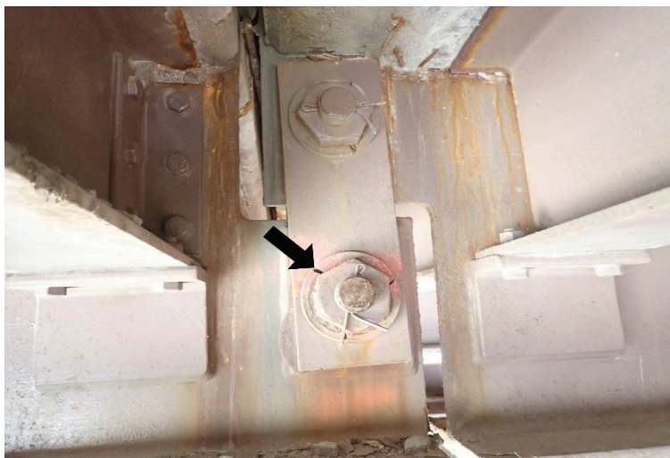
Figure 3-47—Broken spacer washers (arrow) in a pin and hanger connection
