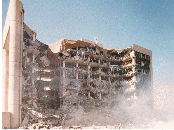
Figure 2. Remains of the Murrah Building after blast-induced progressive collapse
