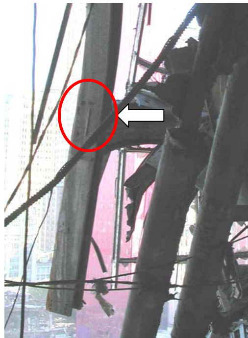
Figure 10. Failed beam-column connection in Deutsche Bank Building
