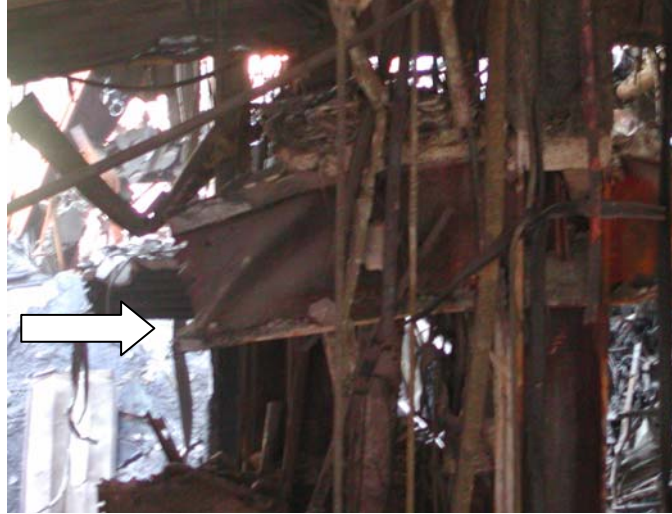
Figure 11. Failed bolted high strength shear connection in World Trade Center 5
