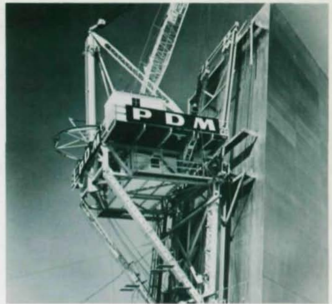
Stifleg derrick rides on steel tracks attached to extrados face of the arch leg.
