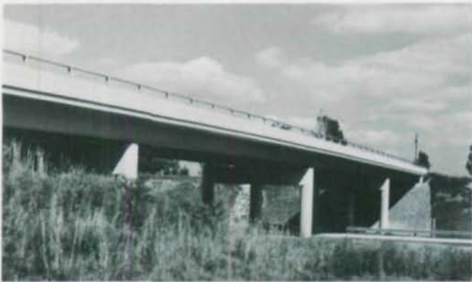
AWARD OF MERIT – HIGHWAY GRADE SEPARATION Interstate 71 Under Gravel Pit Rd., Median County, Ohio Designer: J. E. Greiner Company Owner: State of Ohio, Department of Highways Fabricator: The Burger Iron Company General Contractor: The Harry Miller Excv. Co. & National Engineering & Contracting Co.
