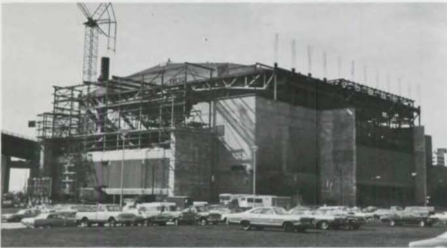
Existing steel is extended upward, then roof is raised to new position.
