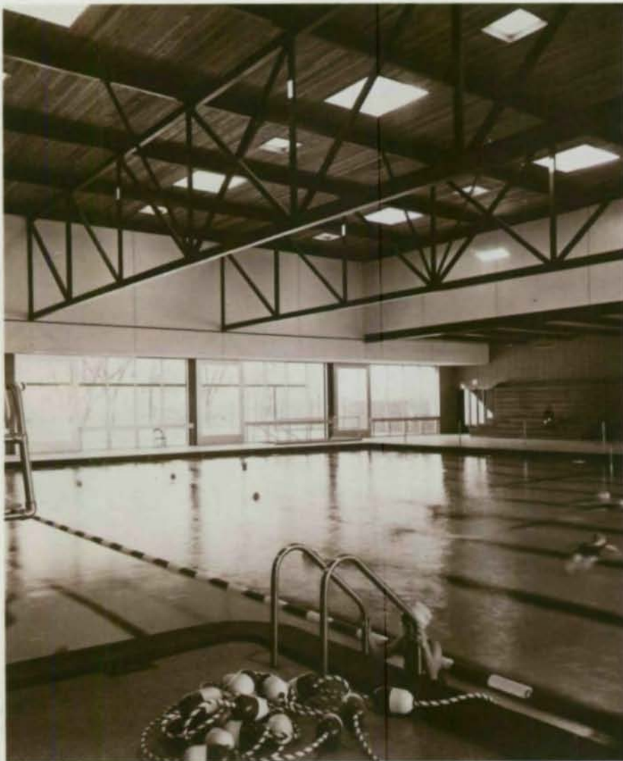
Below: The pool area features welded tubular trusses protected against chlorine and water vapors.
