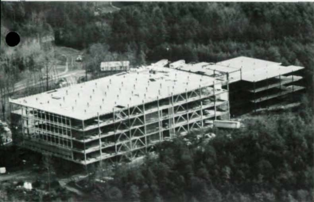
Southern Bell had their corporate data center six months early, thanks to steel-framed construction. Column stubs (top, r.) provide for vertical expansion. Completed structure in heavily wooded site (r.).
