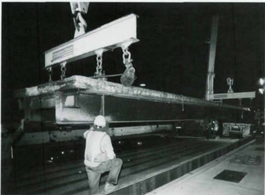
Huge new deck section drops into place (top) during all-night operations. Disintegrating sections (bott.) come out in complex operation.
