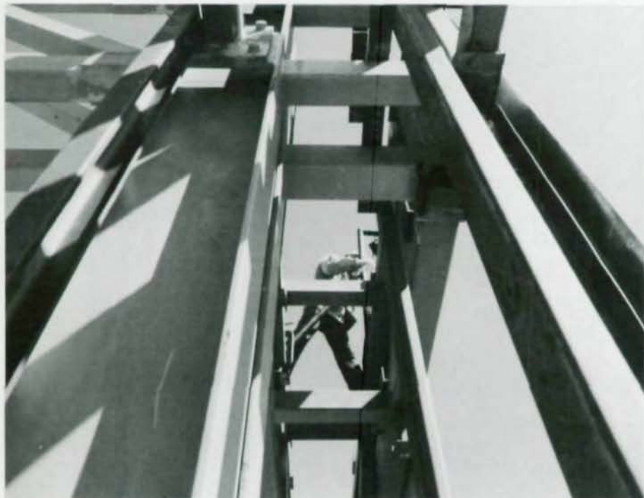
Ozark's concourse was designed to accommodate people-mover above roof (top). Steel-framed project was split into separate bids to speed completion.
