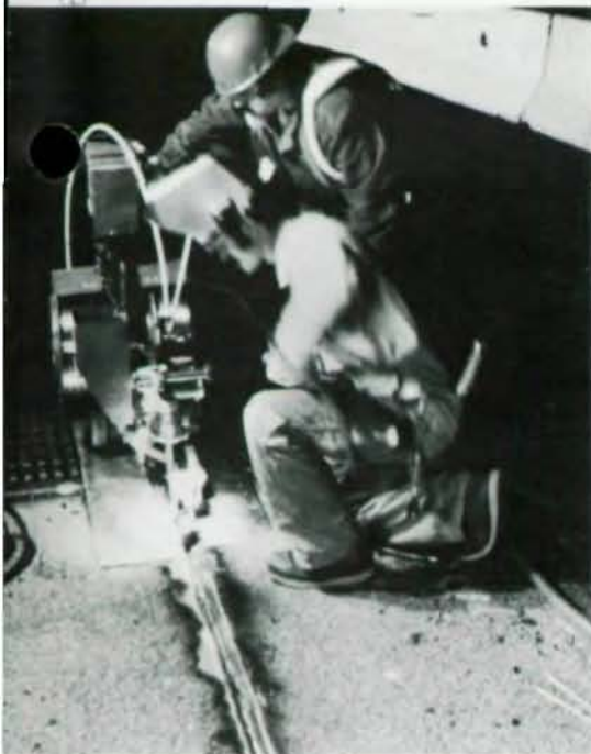
Deck plates were fabricated from 5/8-in. steel plate. Sections were S.A.W-welded on site.
