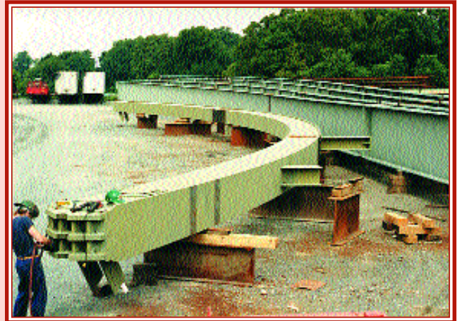
Putting the finishing touches on a weld at the base of a curved box girder.
