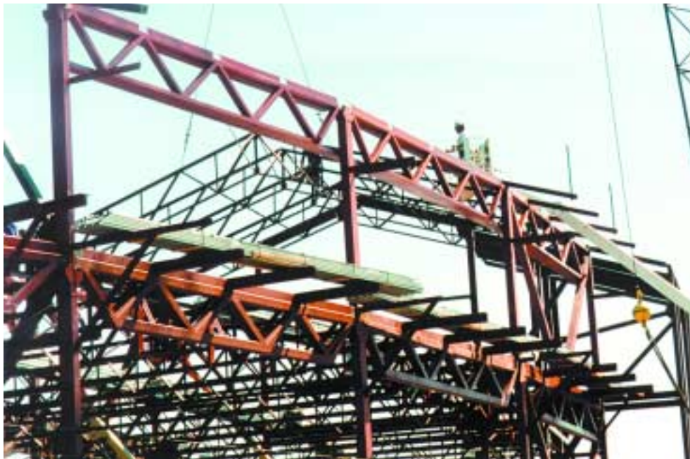
Tube steel girder trusses span along circumference of the building, with joist top chords extending to form exterior walkways.
