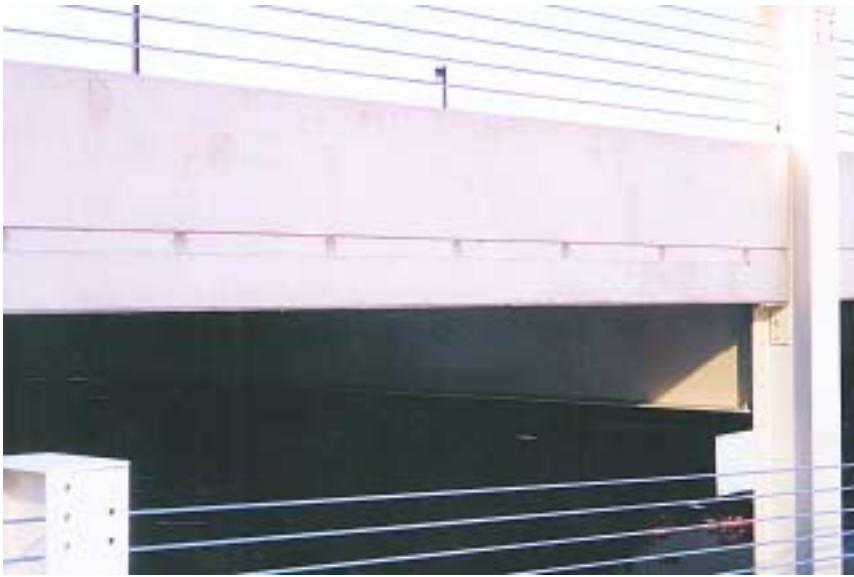
Close up of the P/T anchors showing how the deck, the P/C panels and the steel columns work in a composite manner
