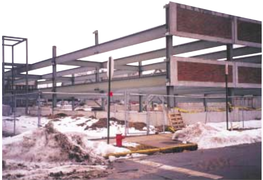
A view of the partially erected steel frame with the P/C concrete panels placed at the exterior for a façade treatment. Note the composite studs affixed to the top of the beams to tie in the concrete deck.
