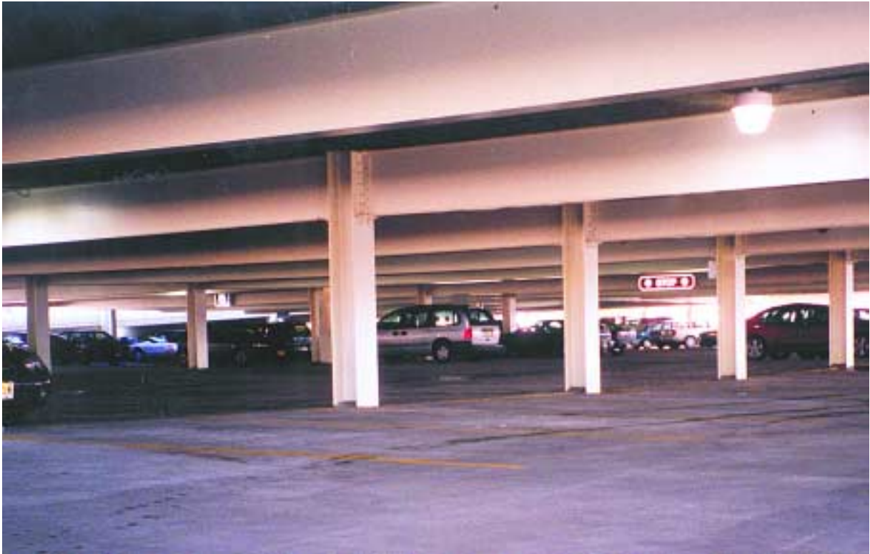
An interior view shows the openness created by the steel framing system. Also note the large deck area free of joints and cracks.
