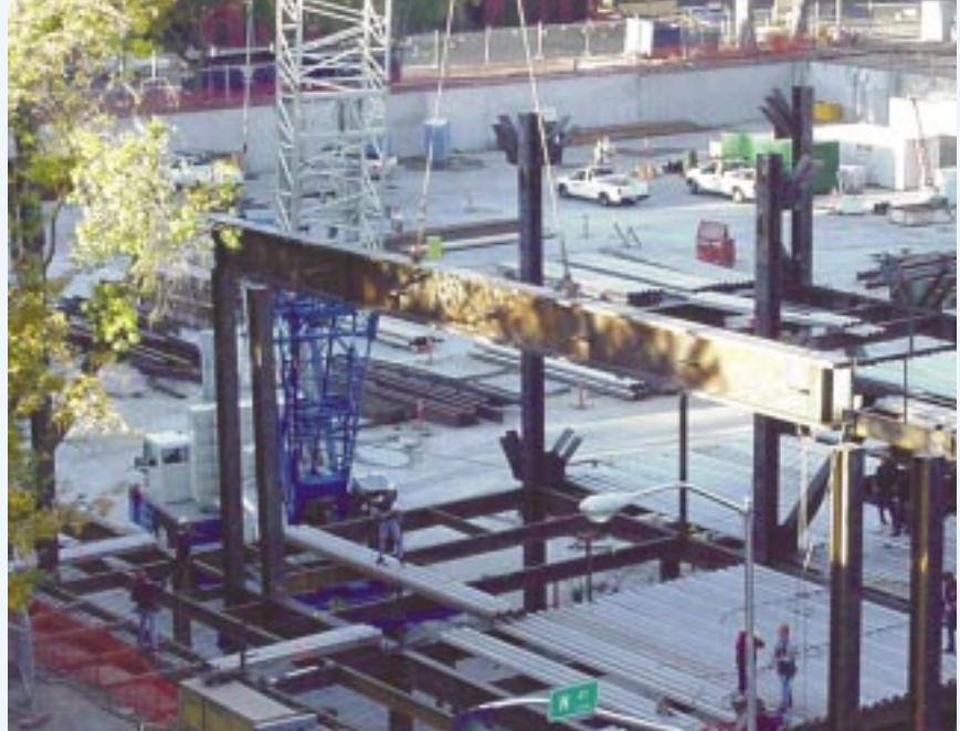
A 46"-deep plate girder spans 65'-0" over the main lobby to provide a column-free space.
