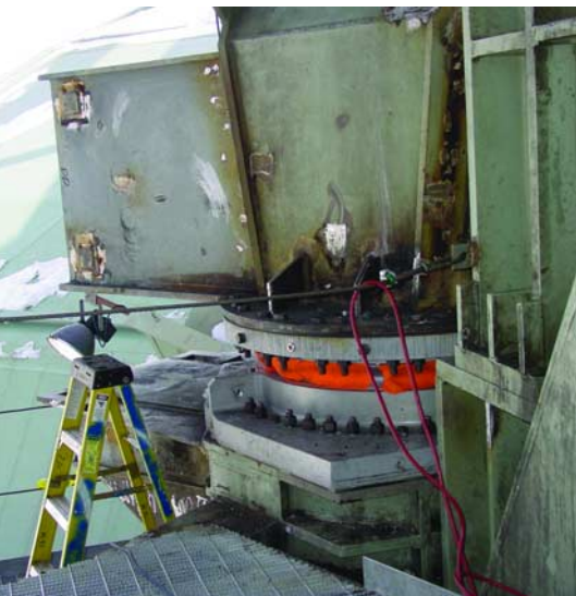
Above: The original bearings were approximately 5' in diameter. Note the jacking bracket (left in photo) attached to the base of the roof-panel frame.
