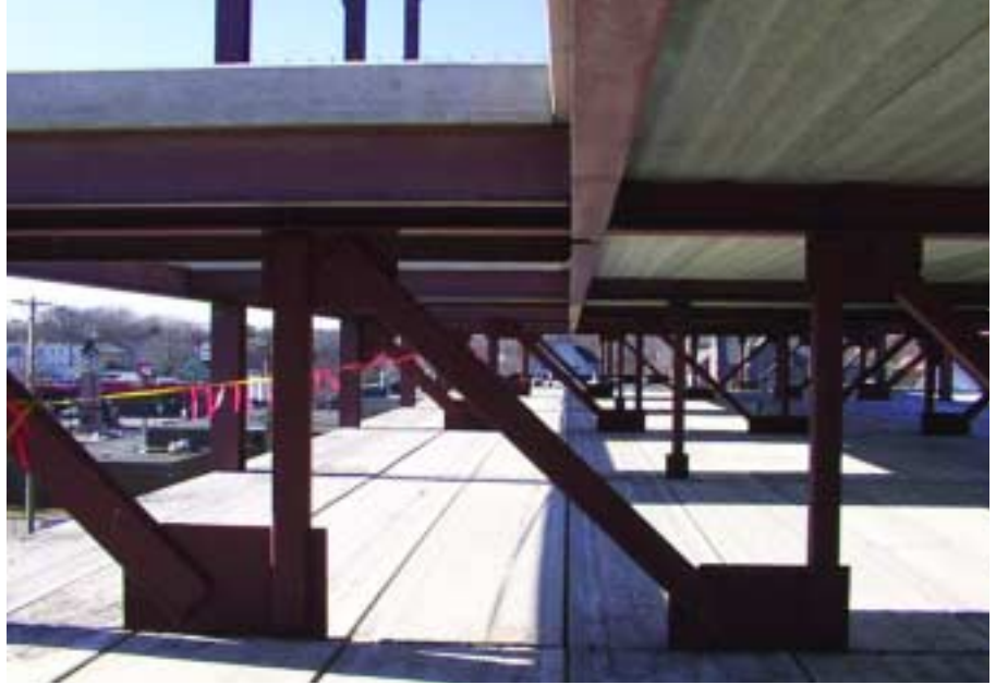
The Legacy Towers' mezzanine loft approach is probably the first of its kind for staggered-truss construction. At each mezzanine floor, the pre-cast concrete floor planks are removed within the interior of the floor plan. This allows each apartment to have a two-level occupancy, where tenants access the mezzanine from their main floor via staircases.
