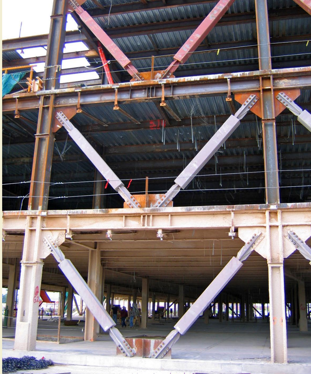
Above: Many of the BRBF columns were jumbo shapes. The BRBF design procedure requires the column to have the strength to resist the vertical component of the expected yield strength of each brace in the frame. Photo courtesy Reaveley Engineers & Associates, Inc.
