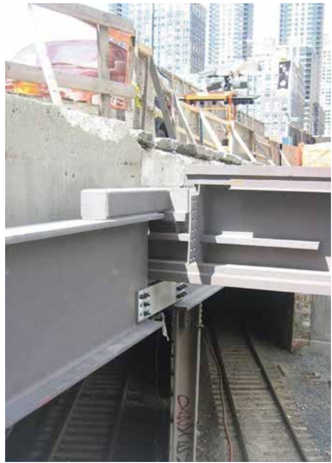
▲ Careful detailing at the train tunnel was required to isolate members supporting the precast tunnel enclosure from the main building structure.
