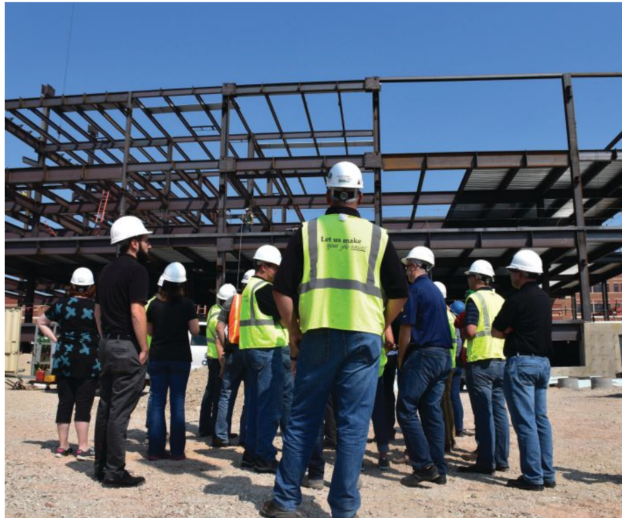
above: SteelDay is a great opportunity for people to visit construction project sites and get an up-close look at how steel framing comes together in the field.
