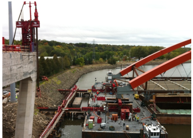
Figure 17: South skid operation
