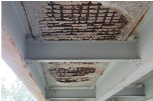
Figure 3: Deterioration of Existing Deck
