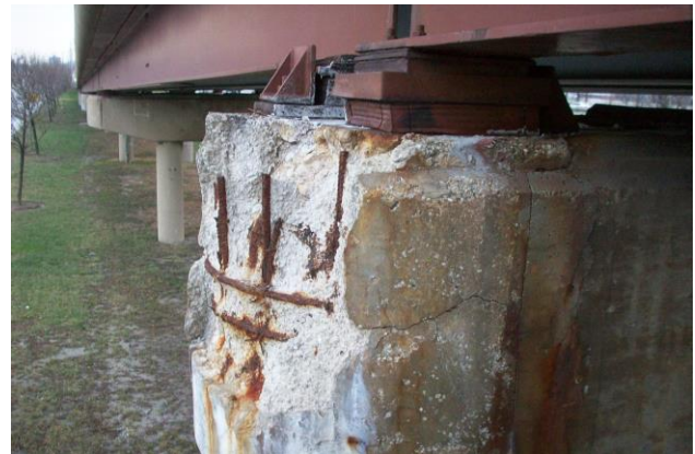
Figure 4: Deterioration of Existing Piers
