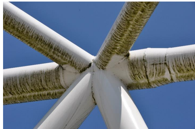
Figure 13 - The drip marks on the underside of the white tubular frame of the AESS truss on this bridge in Vancouver, BC, Canada are the result of less than 2 years of use. The longer this is allowed to accumulate the more difficult it will be to clean. Paint will not adhere properly to the staining if refinishing is chosen in place of cleaning. Photo by author.
