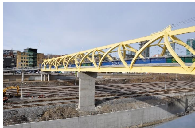
Figure 5 - The Puente de Luz Bridge in Toronto, Canada was erected over a large rail corridor. The fabricator was able to use a night closure of the tracks for the erection. Four cranes were positioned to lift the sections in place and hold until the bolted connections could be made. Tekla drawing by Walters Inc. Photo by author.
