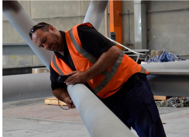
Figure 8 - The thickness of the metalized coating for a bridge in Auckland, New Zealand is being tested in this shop applied application. Metallization is commonly used in New Zealand due to its corrosive marine environment. Photo by author.
