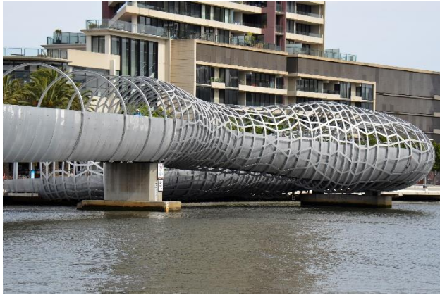
Figure 14 - The Webb Bridge in Melbourne, Australia is suffering from varying levels of deterioration on some of its components. The high level of articulation and the relative thinness of the steel is a challenge for its coating system. Some peeling is occurring. Some of the fasteners are corroding indicating a complete failure of their galvanic finish. The extreme amount of surface area that has resulted from the design, in the corrosive marine environment, makes this bridge difficult to maintain. Photo by author.
