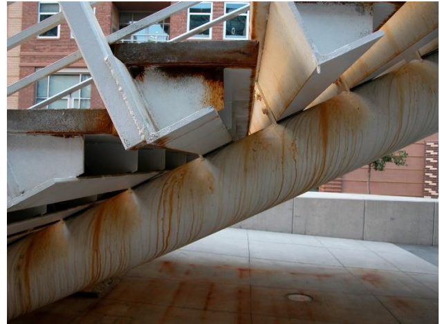
Figure 6 - The stairs on this pedestrian bridge in Denver, Colorado, USA have been improperly designed. The angle components are oriented to collect rather than drain water. The corrosion protection system is inadequate. The local use of de-icing agents was not considered when detailing and designing for corrosion resistance. Photo by author.
