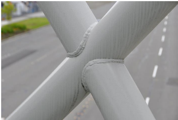
Figure 18 - Simple un-remediated welds were used to connect the elliptical rings that comprise the T. Evans Wyckoff Memorial Bridge . To have ground these welds smooth would have drastically increased the fabrication costs. They are adequately removed from direct sight as to be unnoticeable. Photo by author.
