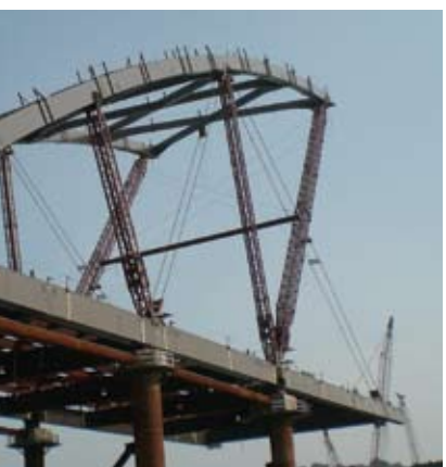
2007: The Blennerhassett Bridge over the Ohio River between West Virginia and Ohio used 30 million lbs. of HPS for its 4,000-ft span.
