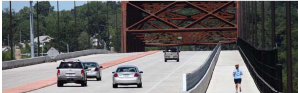
▲ (Top) Erection of the Veterans Memorial Bridge utilized temporary bents at L2' and L6.
