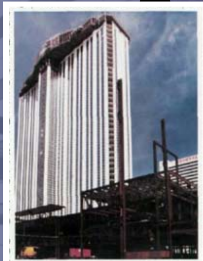
1986: The staggered truss system makes a comeback and is used on the 40-story Resorts International hotel in Atlantic City.
