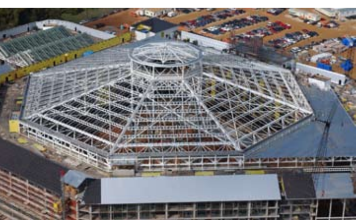
2003: The Gaylord Texan featured cellular steel beams—and will play host to NASCC: The Steel Conference in 2012.
