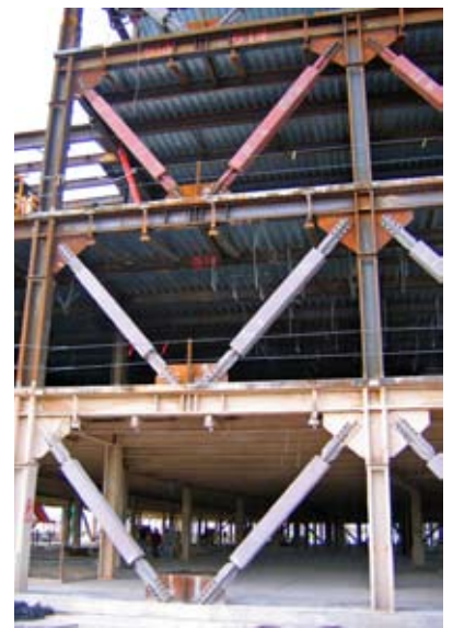
2005: Buckling Restrained Braced Frames (BRBF) became very popular later in the decade. Shown is an early example at the Intermountain Medical Center in Murray, Utah.
