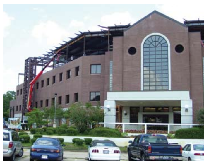
2008: Southpark Hospital in Shreveport, La., remained fully operational while an additional floor was added.
