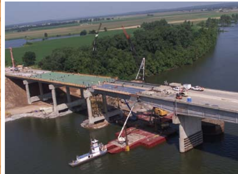
2002: After a pair of errant barges knocked down the I-40 bridge at Weber Falls in Oklahoma, the steel industry mobilized to get a new bridge up and open in just two months.
