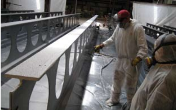
2009: Shop-applied intumescent fire protection cuts the construction schedule on the the BJC Institute of Health in St. Louis.
