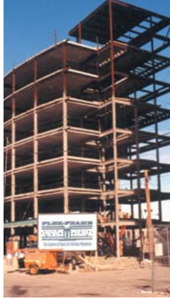
2000: A new system using concrete plank atop a grid of asymmetric steel members is used on a new Drexel University dormitory building. The result is low-floor-to-floor heights and incredibly rapid construction. The system ultimately leads to the development of the increasingly popular Girder-Slab® System.
