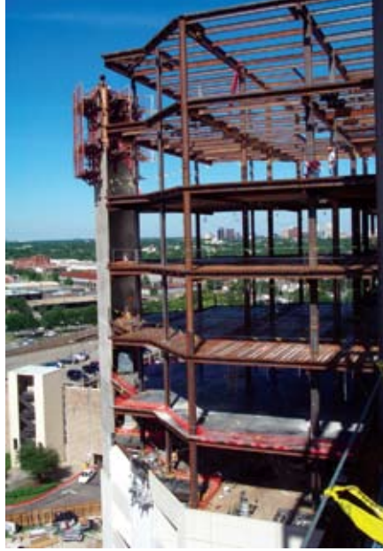
2003: For the Dallas Children's Medical Center, steel was the answer for adding six stories to the existing concrete structure.
