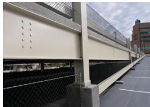
2008: A steel framed, post-tensioned slab system proved economical for a parking structure at Ruby Memorial Hospital in Morgantown, W.Va.
