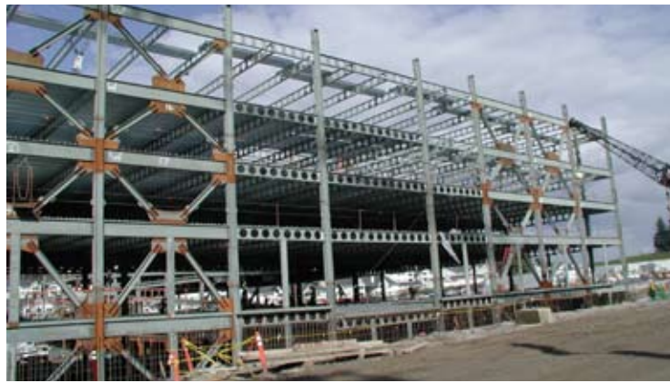
2005: The parking structure for the Legacy Salmon Creek Hospital in Vancouver, Wash., is an early example of the SmartBeam™ system in a parking structure.
