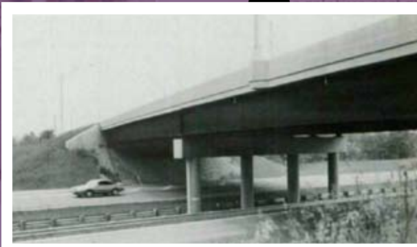
1990: The bridge on State Route 739 over US33 in Union County, Ohio, was an early adopter of integral abutments.
