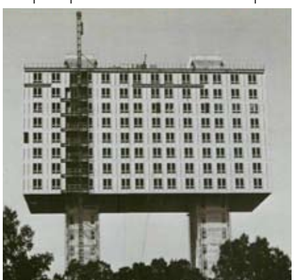
1975: The Russian Residence in New York City utilizes a slip form concrete core and a unique top-down construction technique.
