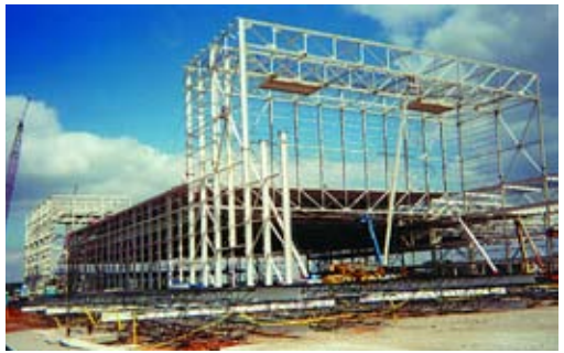
1999: It only took 26 months from the start of design to the completion of construction on the 1.5-million-sq.-ft Boeing Rocket Booster facility in Decatur, Ga.
