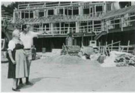
1984: Maria von Trapp (yes, from the Sound of Music) looks over the steel framing for the new von Trapp Family Lodge in Stowe, Vt.
