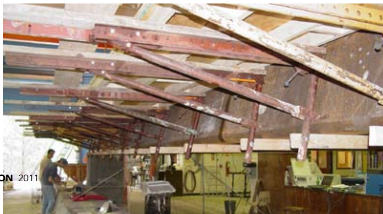
2009: Folded plate girder bridge systems have the potential to revolutionize the short-span bridge market.
