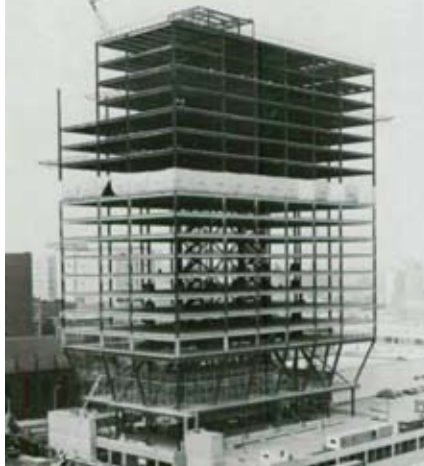
1981: One Corporate Center in Hartford, Conn., demonstrates the growing trend toward vertical expansions as it rises 16 stories on top of an existing building.
