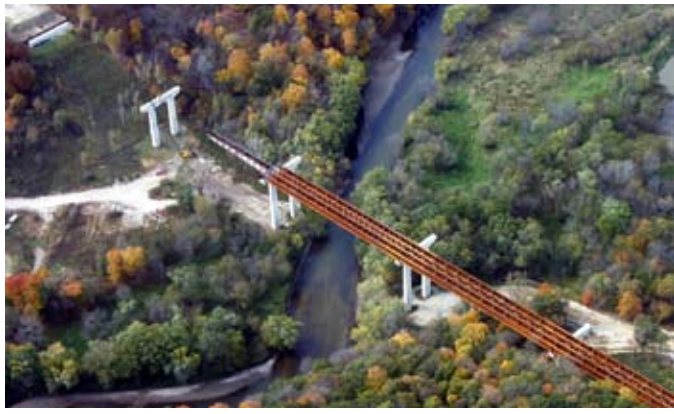
2004: The US20 bridge over the Iowa River is the first in the U.S. to use the incremental launch method for erecting an I-girder bridge.
