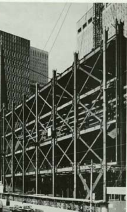
1970: The designers of the Bell Telephone Building in Pittsburgh use 100 ksi steel for its X-bracing.
