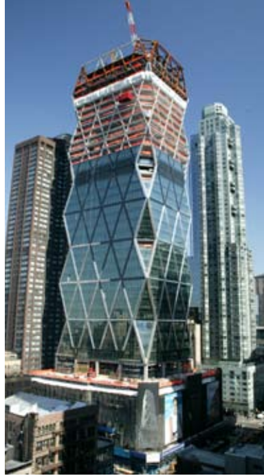
2006: A diagrid steel frame gained attention for the 46-story Hearst Building in New York City.
