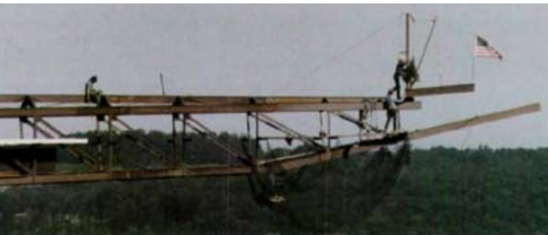
1988: A tube of wide flange sections creates an "infinity room" and a new tourist attraction at the House on the Rock in Spring Green, Wis.
