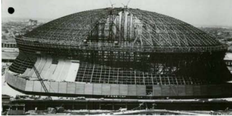
1976: The Louisiana Superdome is the world's largest fixed domed structure and its steel frame covers a 13-acre expanse.
