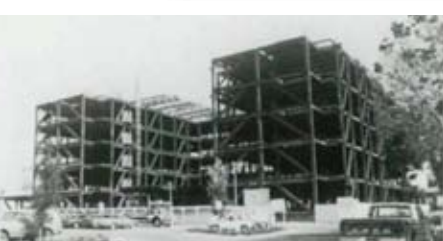
1980: The O'Connor Hospital in San Jose, Calif., is an early use of eccentric braced frames for seismic design.
